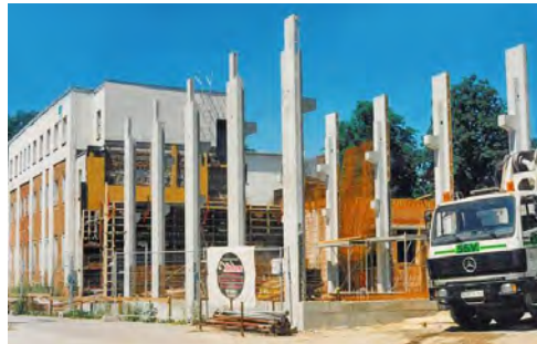
1995: Construction work on the technology center for the Fraunhofer CAM; today, it houses the lab for the TITAN electron microscope.
